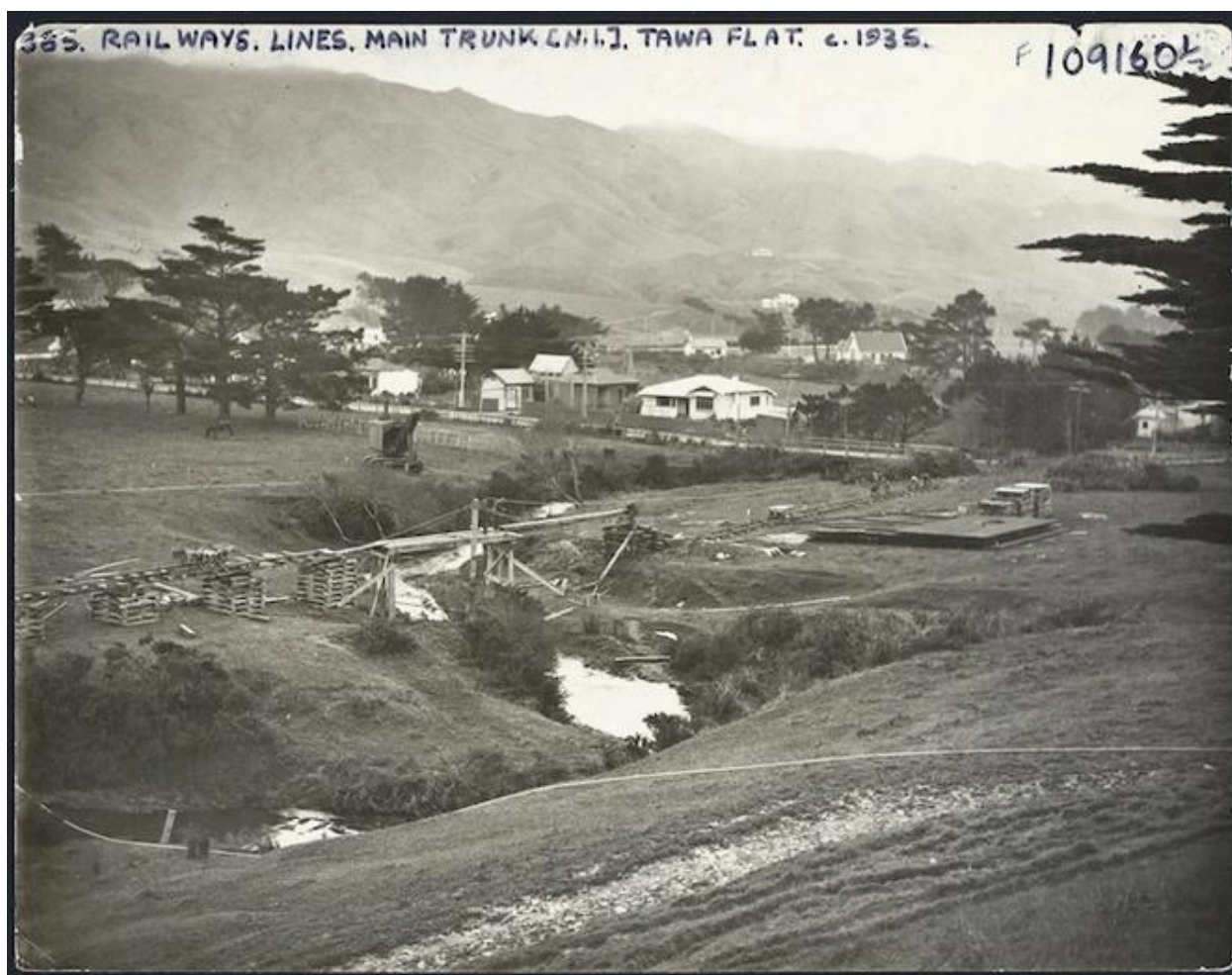
Construction of the main trunk railway... | Items | National Library of New Zealand | National Library of New Zealand Construction of the main trunk railway line, Tawa Flat, Wellington
