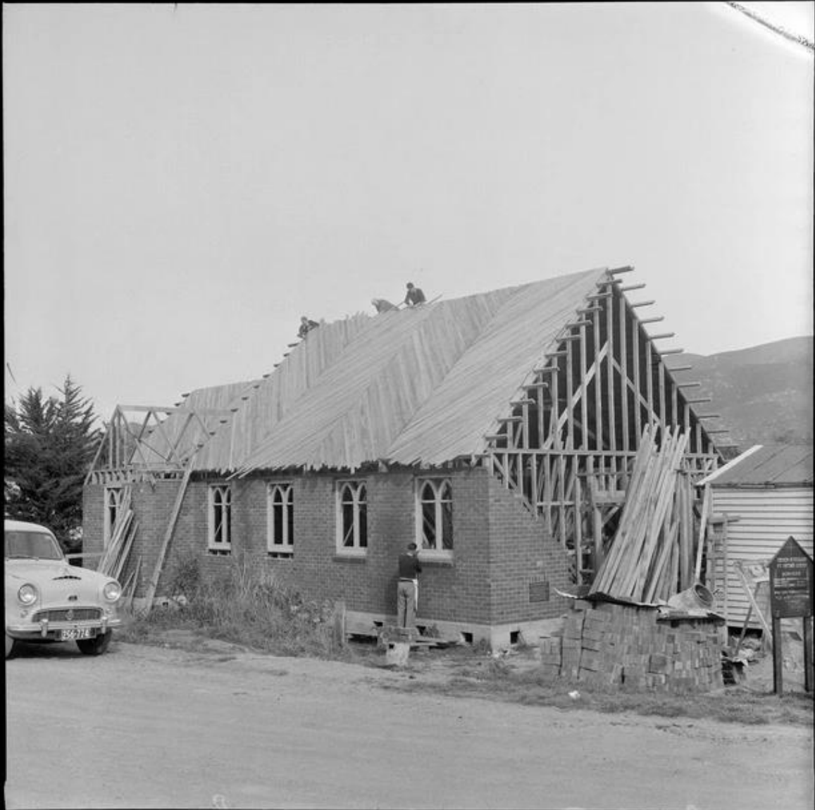
St Peter's Anglican church under cons... | Items | National Library of New Zealand | National Library of New Zealand Date 1957 Reference EP/1957/3475-F Description Photograph taken for the Evening Post newspaper of Wellington by an unidentified staff photographer. Access restrictions Part of Evening post (Newspaper. 1865-2002) :Photographic negatives and prints of the Evening Post newspaper / Negatives of the Evening Post newspaper
