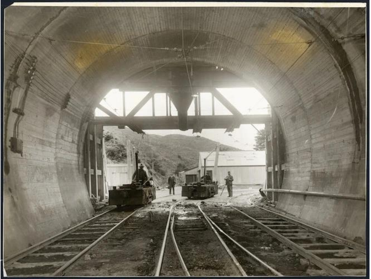
Newly constructed railway tunnel on t... | Items | National Library of New Zealand | National Library of New Zealand Date [ca 3 Nov 1933] Reference PAColl-9150-08 Description Looking out from a newly constructed railway tunnel on the main trunk line at Tawa Flat, Wellington. Shows the view from No 4 portal, the Glenside end of the Tawa Flat deviation tunnels, showing two of the electric engines used for the haulage of spoil and construction material. Photograph taken circa 3 November 1933 by an unidentified photographer. Other - Note on back of print read: "Wgtn Studio Photo" Cataloguer is unsure what this means. Possibly not an Evening Post staff photograph. Part of Evening post (Newspaper. 1865-2002) :Photographic negatives and prints of the Evening Post newspaper / Evening Post photographic prints
